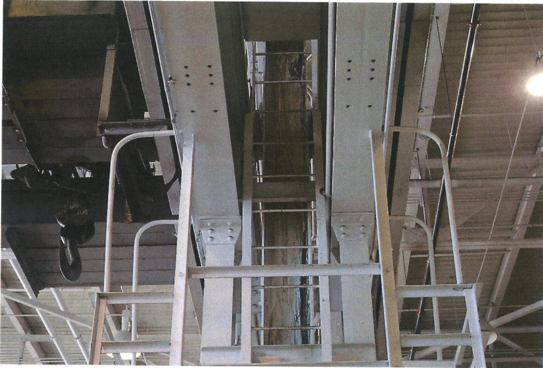
Evidence of water leak on column B3
