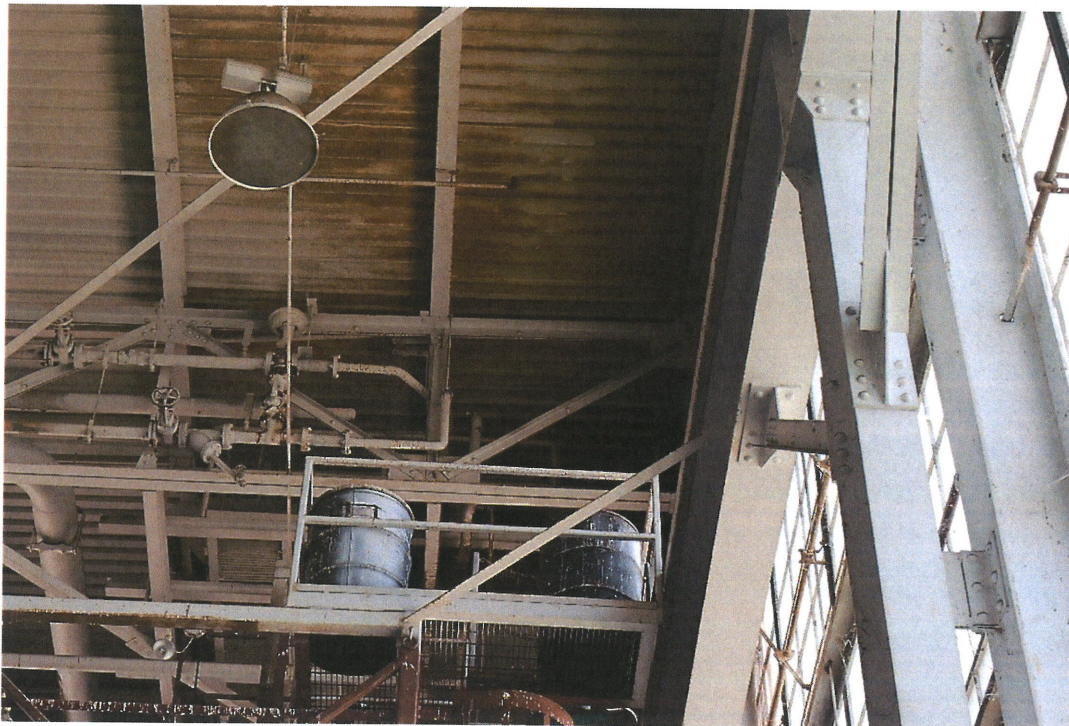
Close view of corrosion
