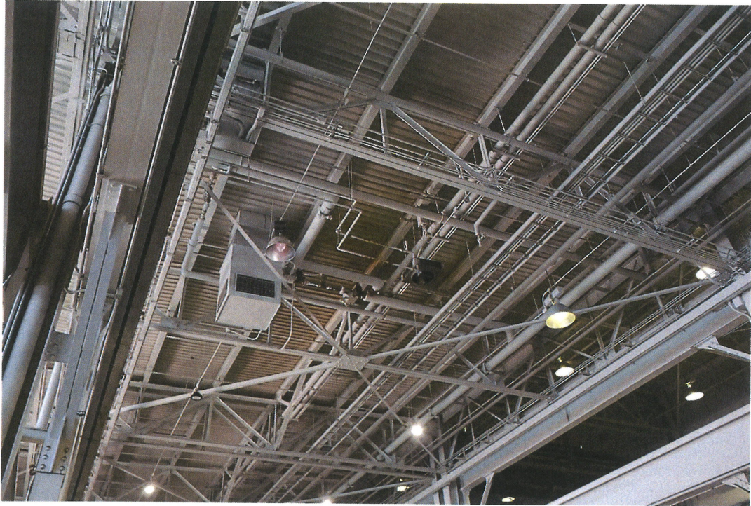
Minor corrosion in roof near column B6
