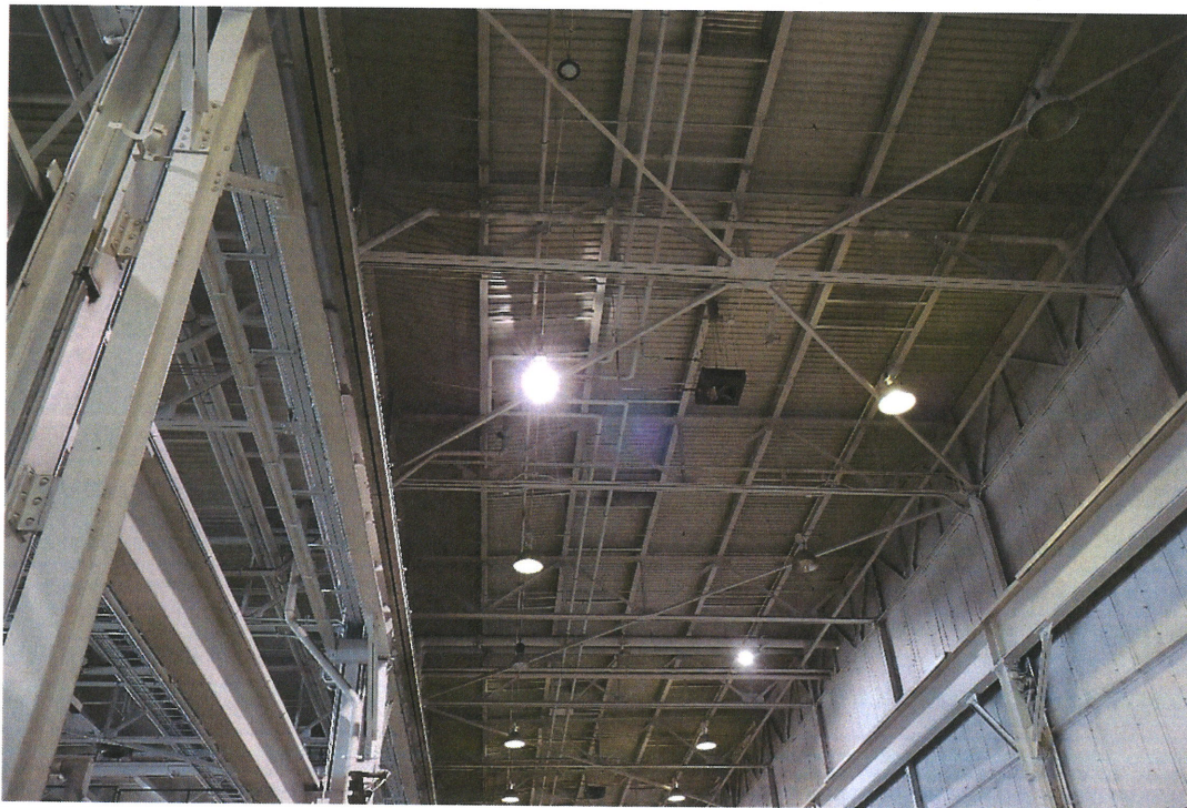
Looking North in Highbay
