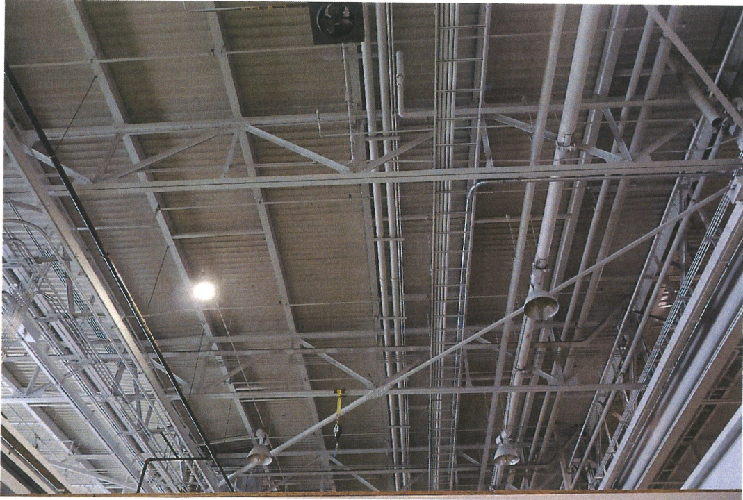
Looking North in Highbay
